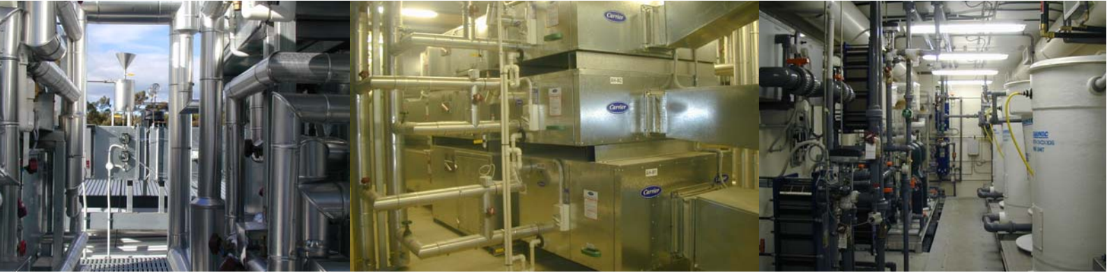
▲ AAD, rooftop AC plant, 4.5 star NABERS rating
